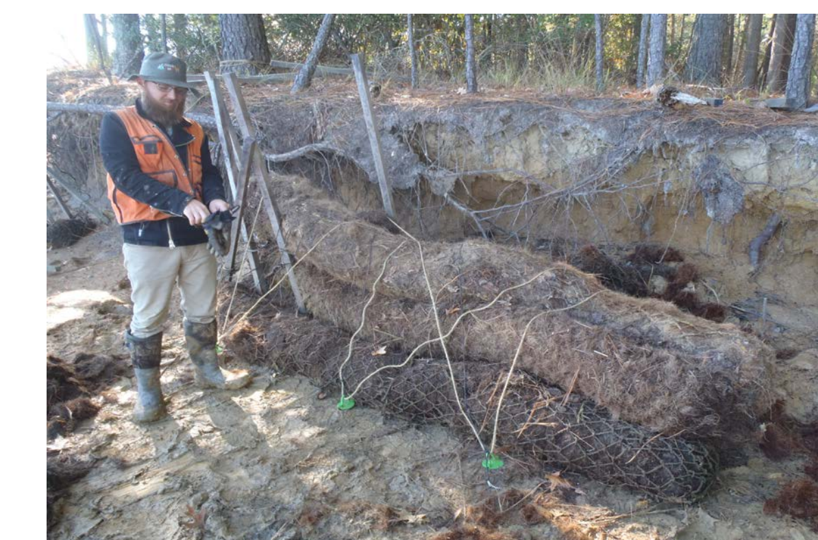
CSU employee William Feltz installs the new metal tent stake anchoring system at site 44NN14.
